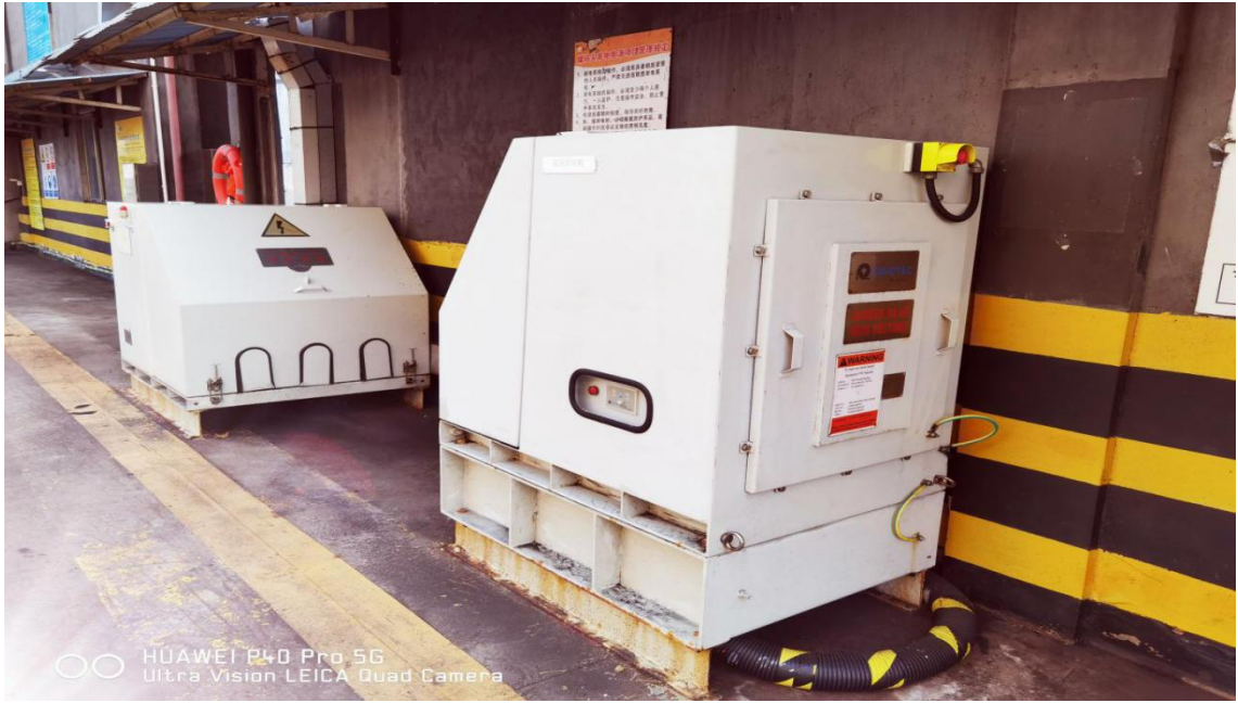
High-voltage socket box and low-voltage socket box
