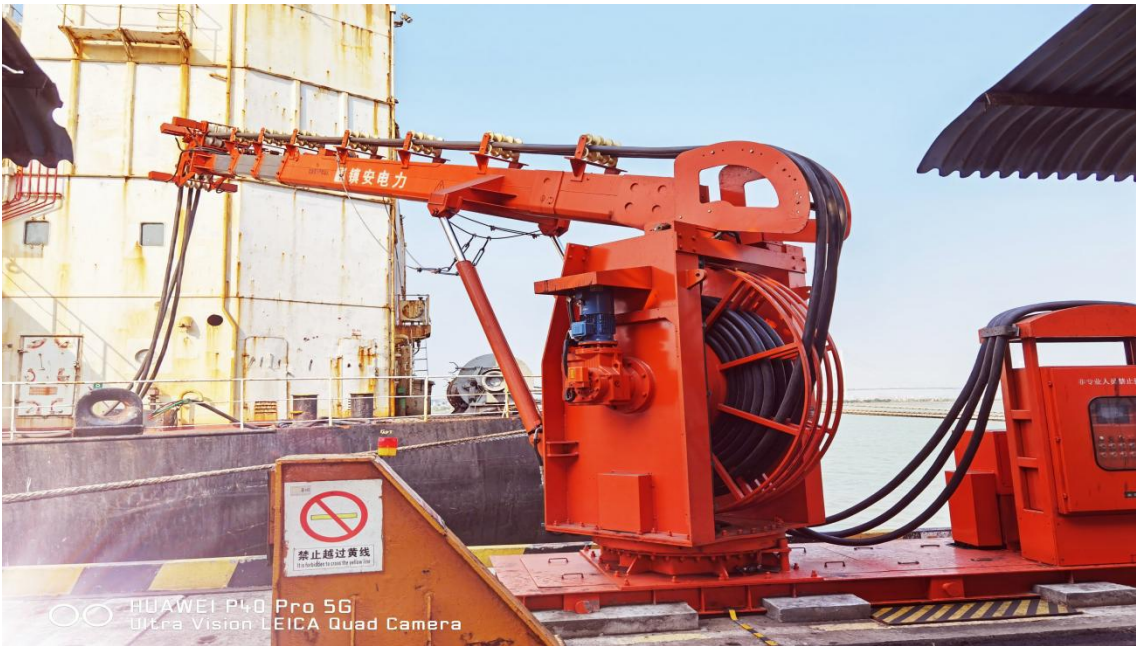
Lifting device of shore power cables
