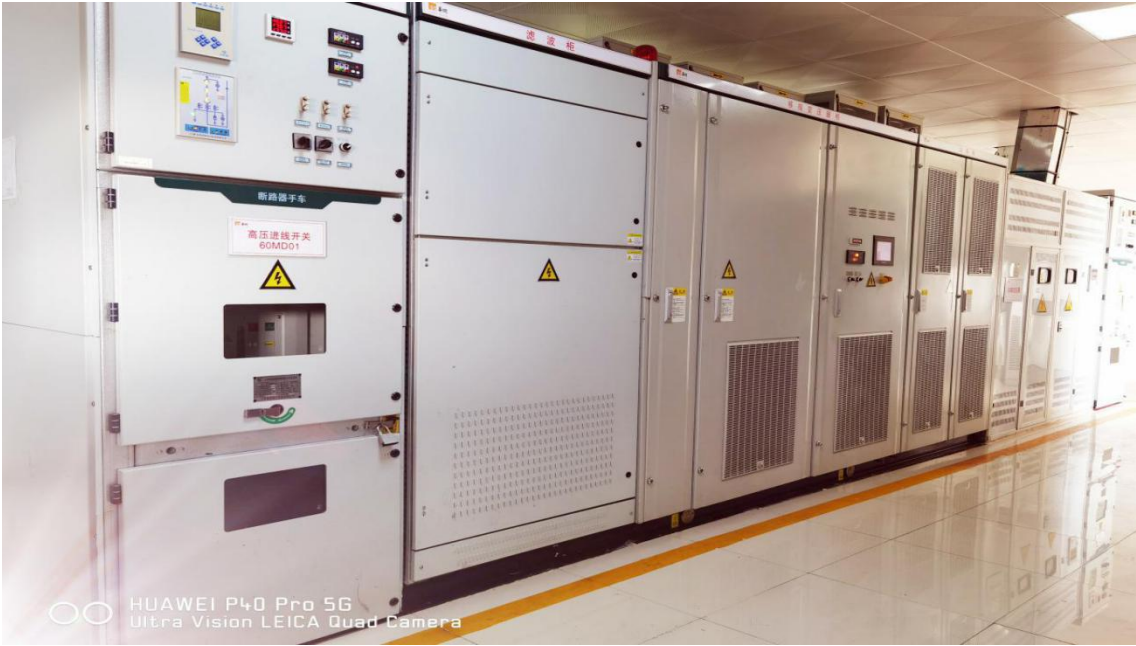
Electricity distribution room of shore power facilities
