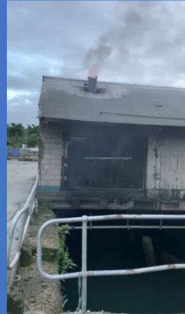
OLD DIESEL INCINERATOR
