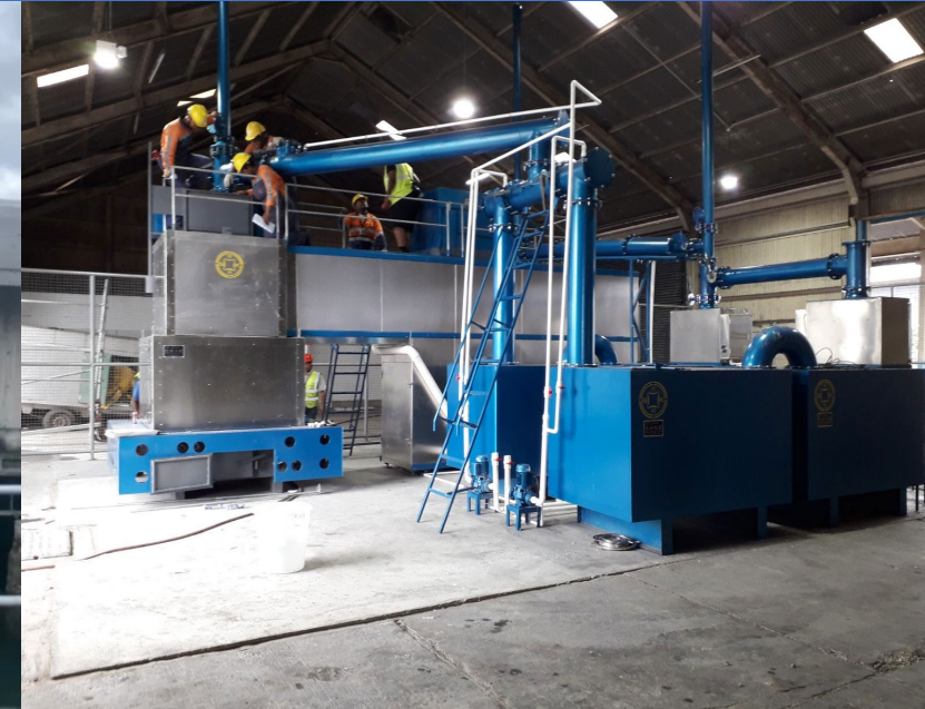
ELECTRIC INCINERATOR AT SUVA PORT
