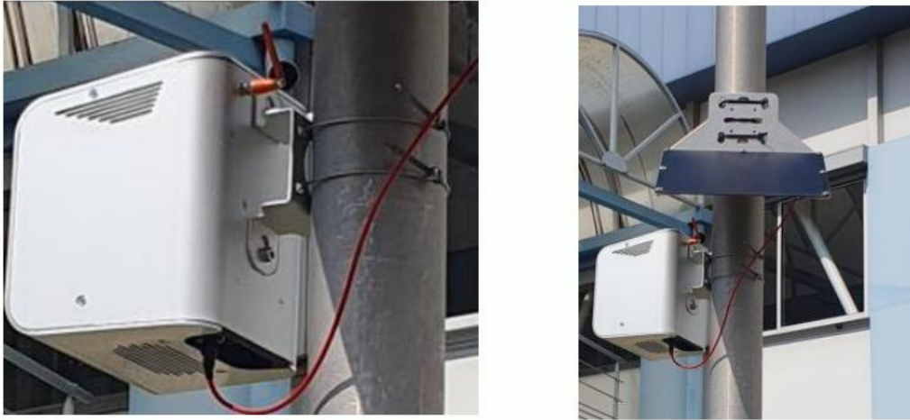
Example of Deployment: Urban infrastructures on lamppost with power supply
