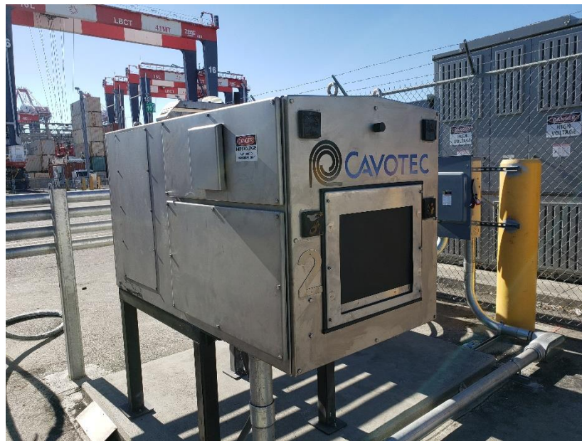
Figure 2: Cavotec SPS Charging System – ITS/POLB
