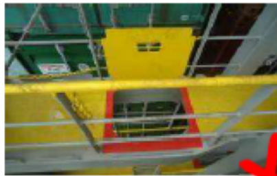
Bridge manhole without safety chains
