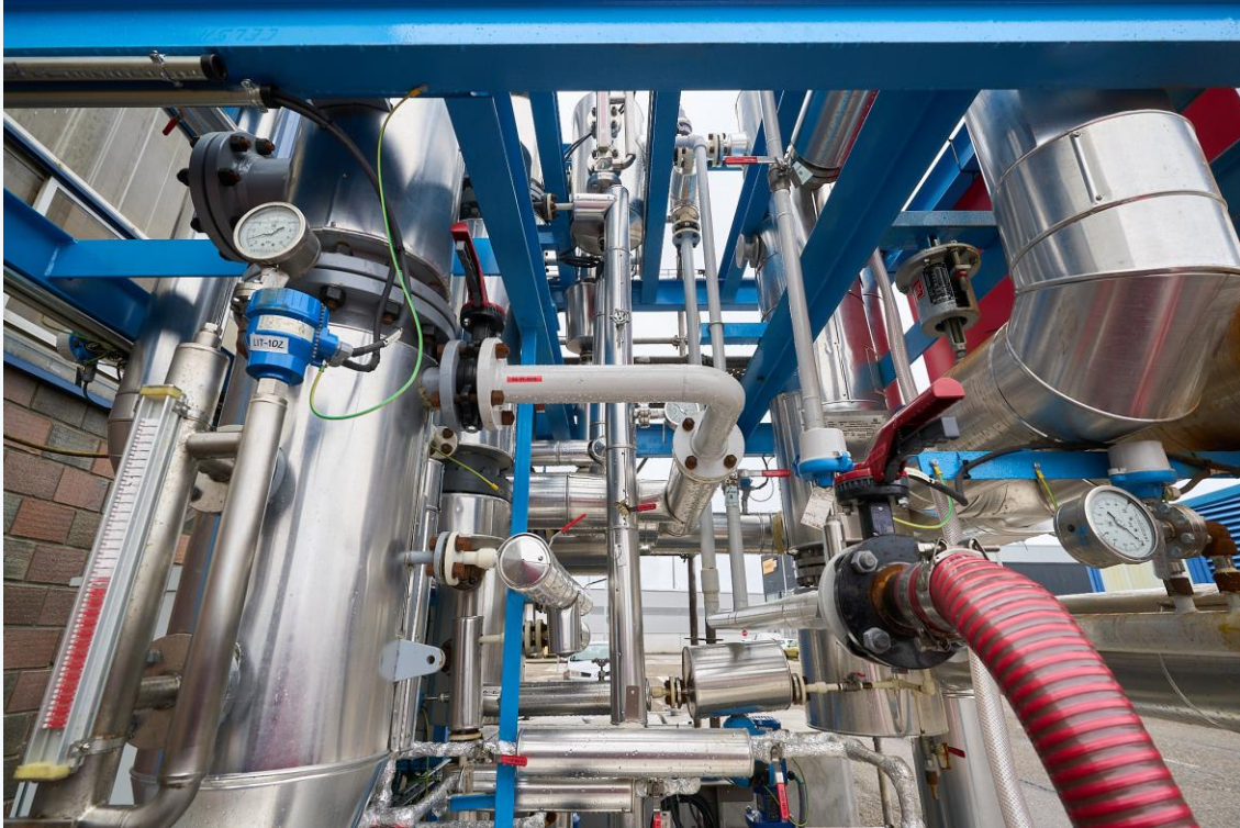
Absorption and regeneration columns
