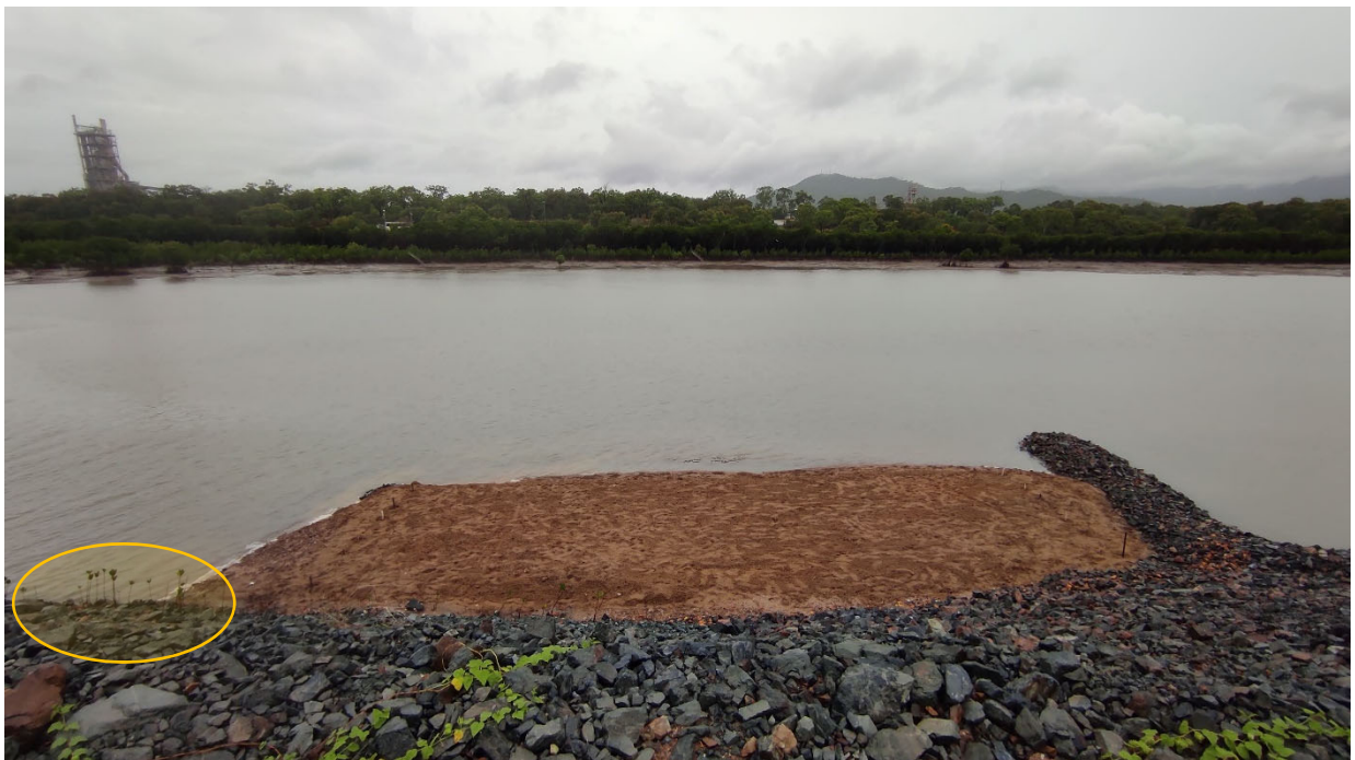
Figure 2: Photo of one of the completed sites, taken in January 2023. In the lower left of the image, along the base of the rock wall, there are some mangrove saplings visible – these and others similar were included in the disturbance estimate submitted as part of the original development application, but were left undisturbed during the construction process.
