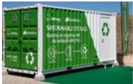
Second life batteries
