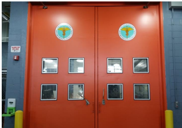
Test cell doors
