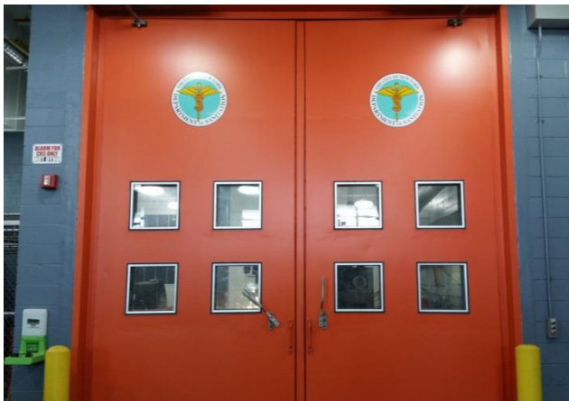
Test cell doors
