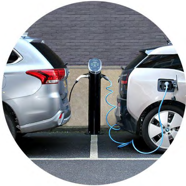
Figure 9—10 An Example 7kW EV charger
