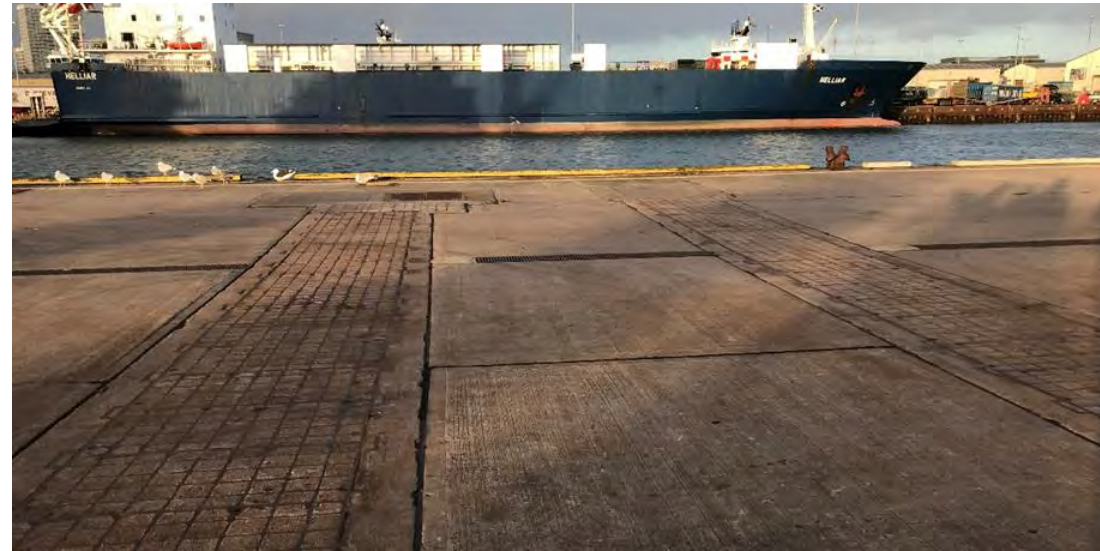
Figure 4—17 Site visit photograph showing concrete service trenches at Albert Quay. It is noted that the trench on the right of the photo has been infilled with concrete and is therefore assumed to be redundant.
