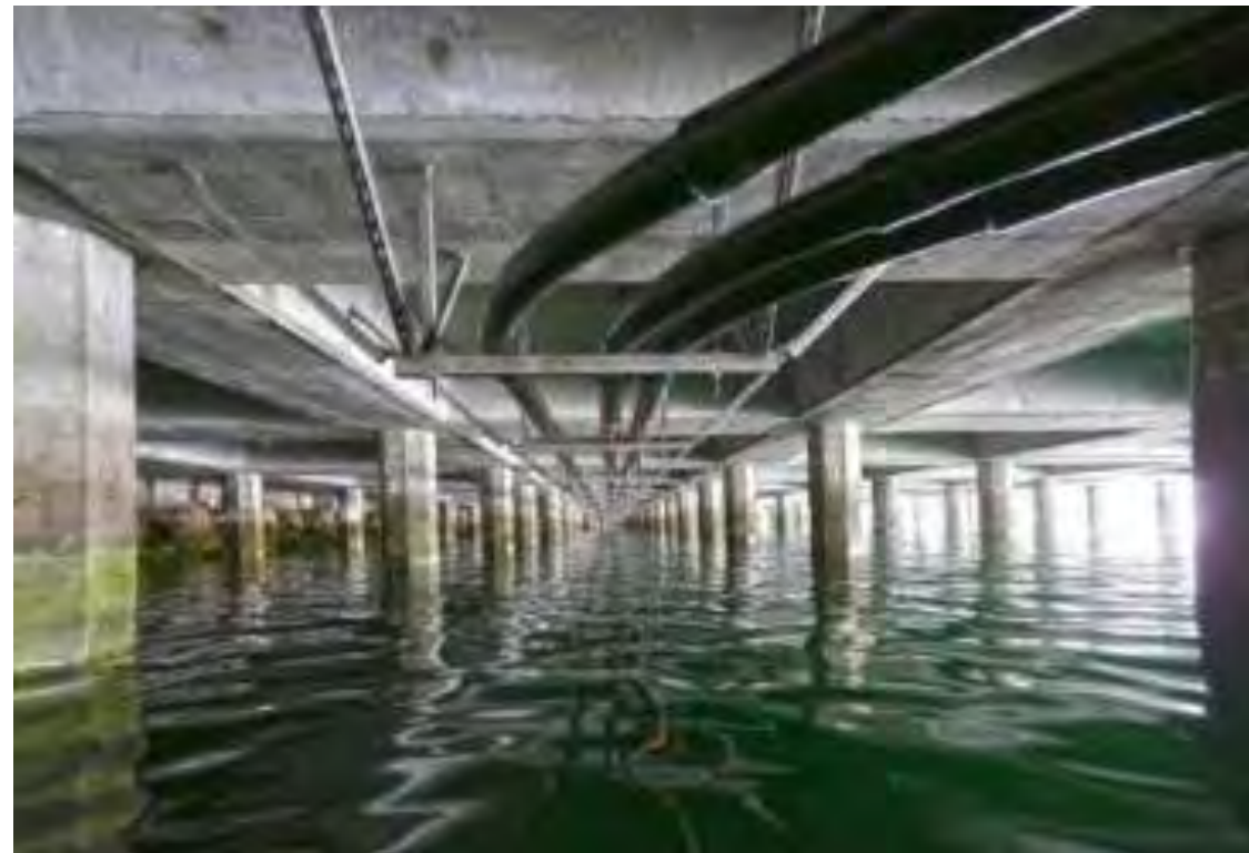
Figure 9—25 Ducted power cables beneath the Port of Long Beach (from EMSA 20 )
