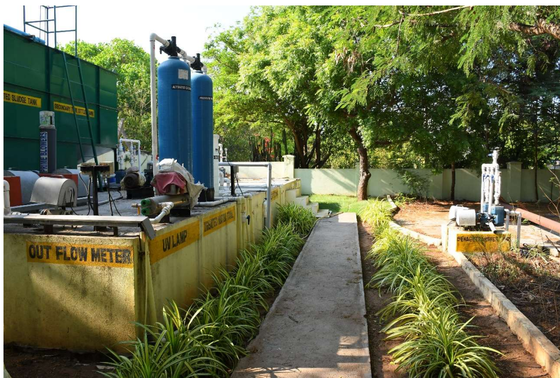
Sewage treatment plant installed: Reuse of water for irrigation purposes with a aim of zero water wastage
