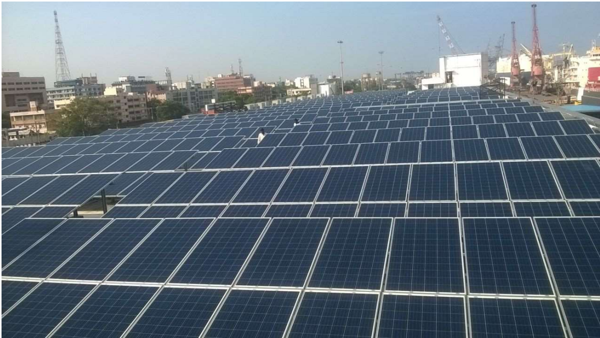
Shifting towards Clean energy: Rooftop solar panel installed in building.
