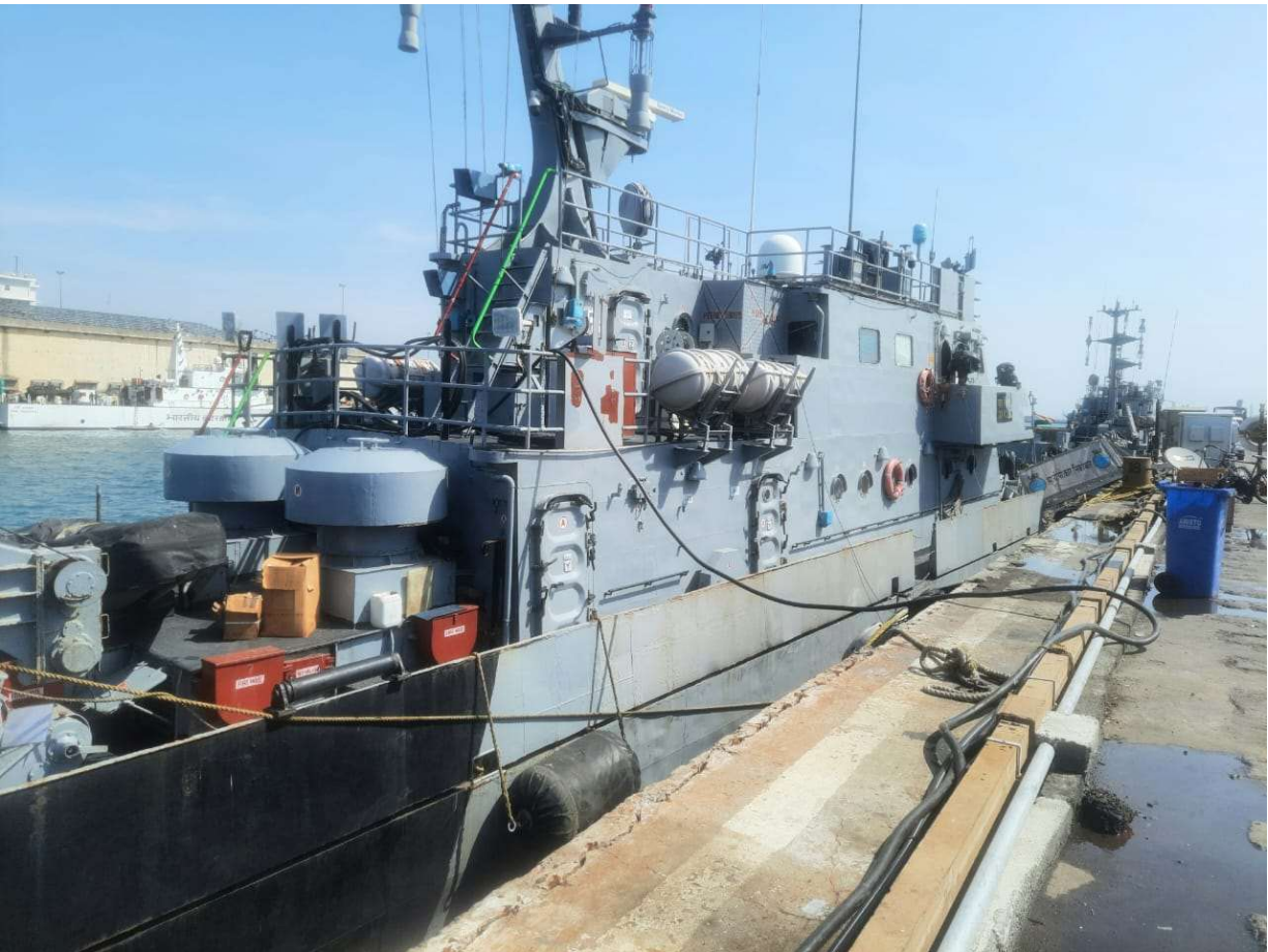
Shore power supply to berthed vessels: Reduction emissions compared to use of diesel engine by vessels
