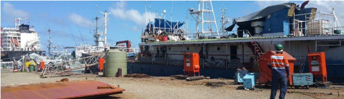
Figure 1 FSHIL has already installed shore power (the orange boxes along the wharf)
