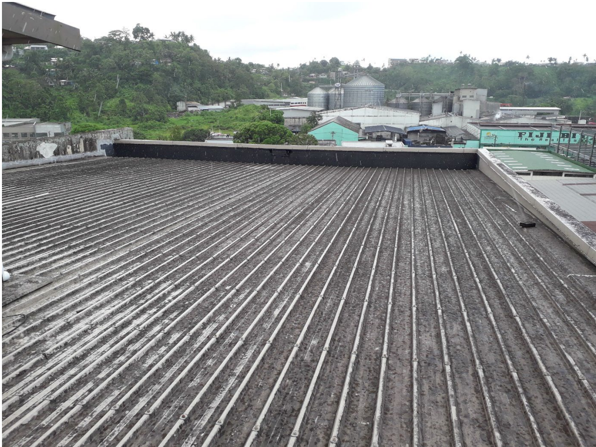
Figure 8 The rooftop of Muaiwalu House, and the rooftop of Muaiwalu waiting area are suited to the installation of solar PV.
