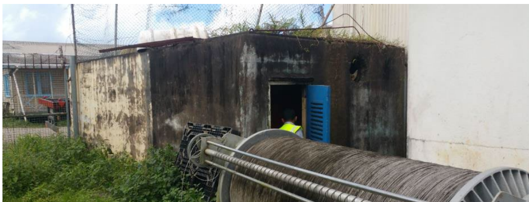
Figure 7 EFL substation supplying Muaiwalu 1. FPCLs meter is inside this substation building
