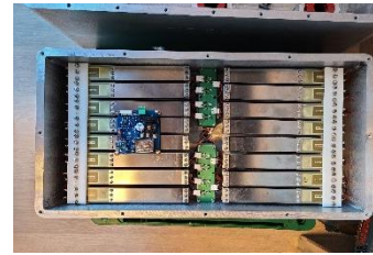
[IoT sensor module installed]
