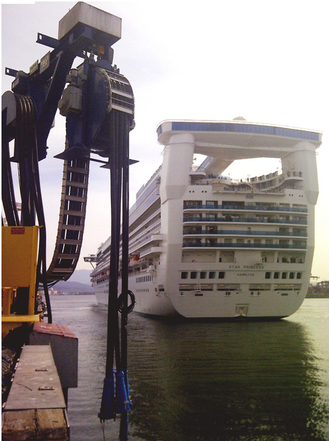
A ship plugging into shore power, which allows large ships to turn off their engines and plug into the electricity grid, cutting emissions. (Port of Vancouver)
