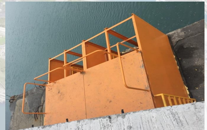
Outfall Sedimentation Control Box
