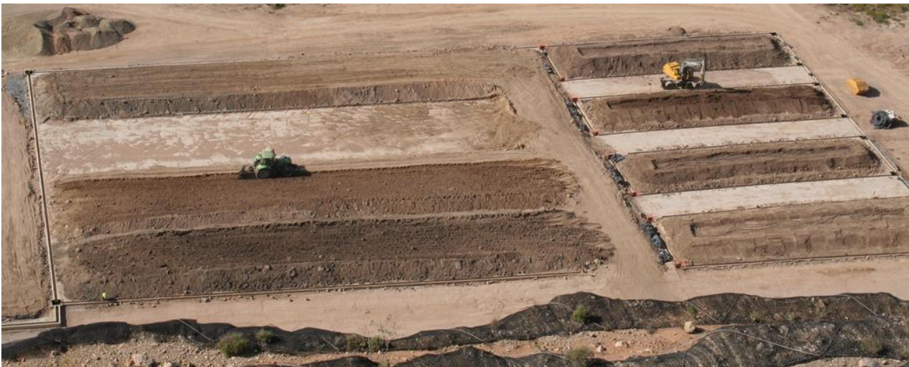
Soil bioremediation plant in Escombreras
