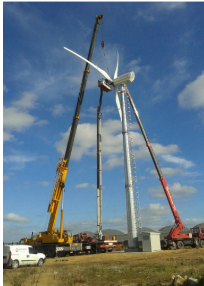
Image: Wind turbines 50 kW
